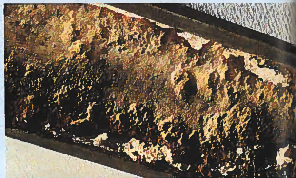
Boiler scale almost fills this hot-water pipe. The deposits consist mostly of \text{CaCO}_3 with some \text{MgCO}_3 .
